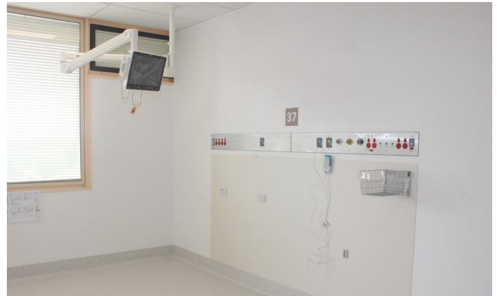
Finishing touches underway: new patient room in the inpatient unit (IPU B6). The new unit opens in April 2018.
